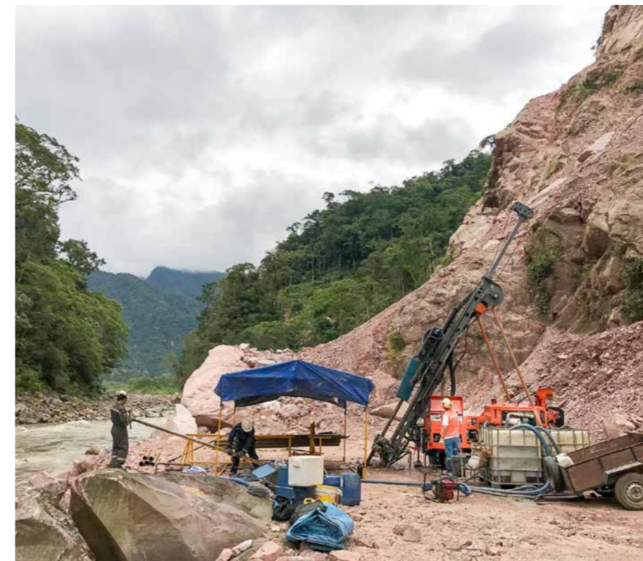
Core drilling in Bolivia. The MK3 has a 74Hp Tier 4 final engine or 111Hp Tier 3 options and rotary head spec of 6000Nm torque and 750 rpm. High speed motors can take this to 1100 rpm.
